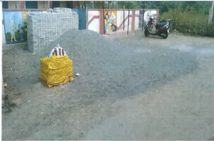
Paver Tiles at Mulliseval School (Before)
