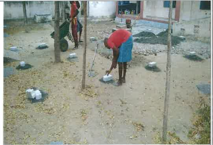
Paver Tiles at Mulliseval School (Before)
